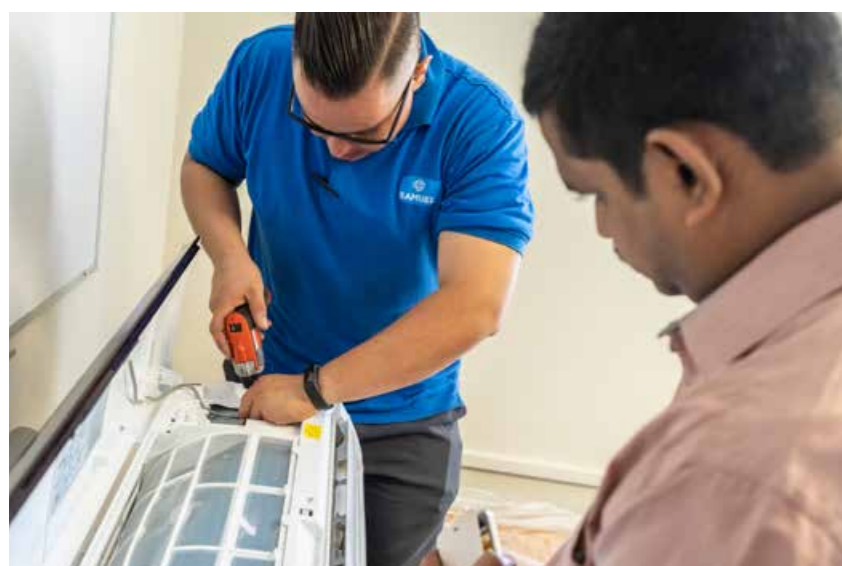
The installed R290 ACs consume at least 20% less electrical energy than conventional reference units installed in the same buildings.
